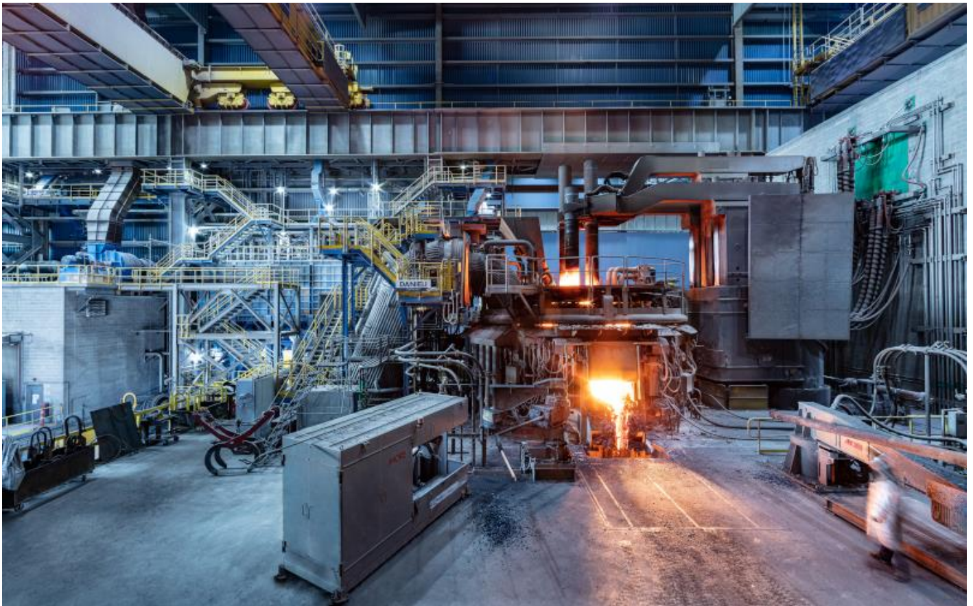
Algoma Steel is installing electric arc furnaces, which will be powered by Ontario's green electrical grid, at its steelmaking operations. Courtesy of Danieli
